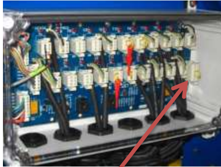
Large Junction Box Right-Side
