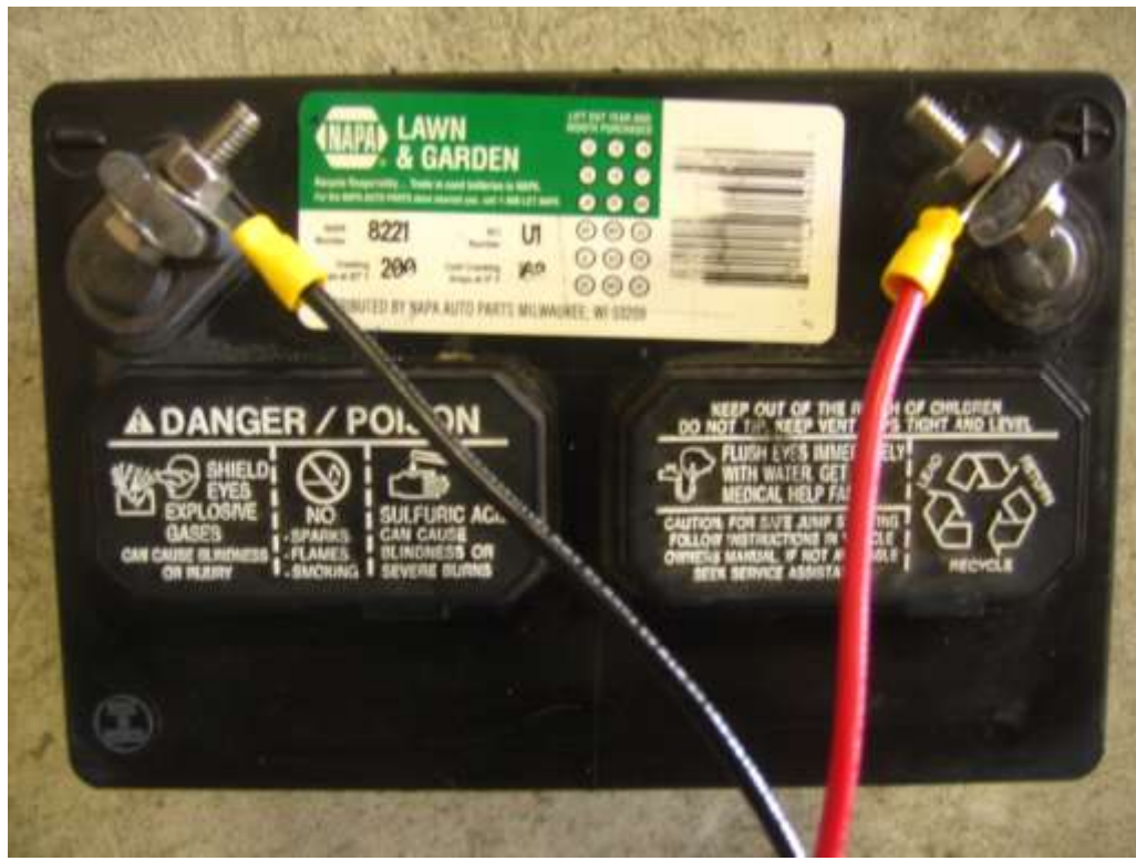
Figure 7: Power Source Cord to Battery.
