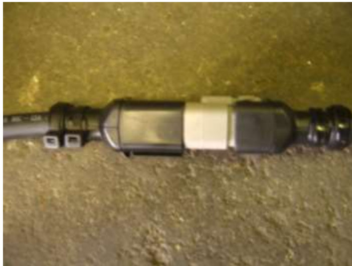
Figure 6. 1. Controller Cord 2 to Junction Box Cord 2; 2. Controller's Power Cord to Power Source Cord (Battery). Single way connections.
