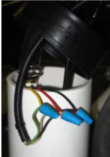
Wiring connection inside of Tube
