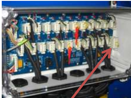
Large Junction Box Right-Side
